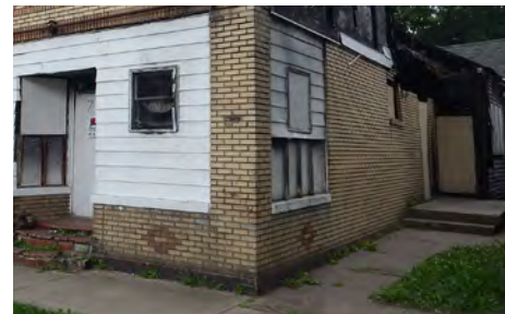
6. Condition and disrepair of building stock
